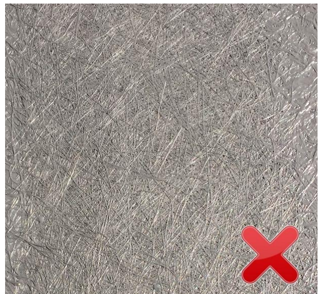
The first coat applied with too little resin or the matting not worked enough, with fibres still straight in appearance
