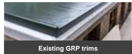
Flaking top coat
